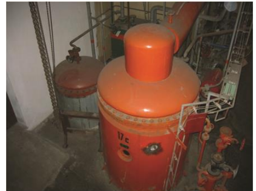
Old evaporator (heater and separator)
