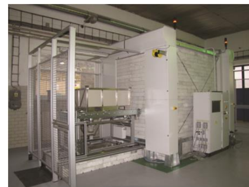
Measuring device for release of waste into the environment
